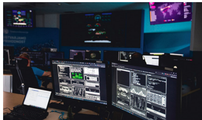
Fig 2: Cyber Security Operations Centre of Telekom Slovenije
